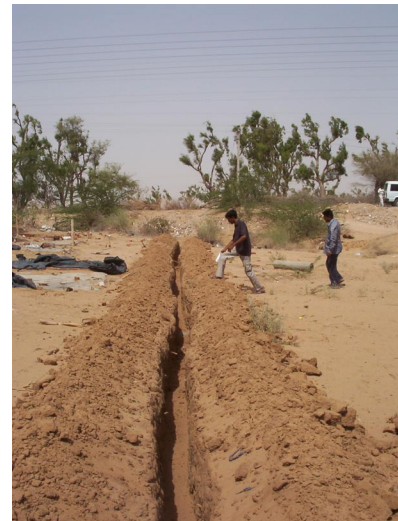
Water line under construction, running E-W along N edge of site; dismantled laborers quarters shown at upper left.
